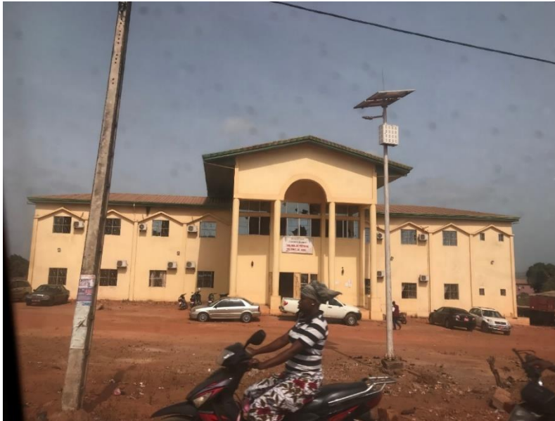
Administrative building in Boké town with windows smashed in February 2018 by youths protesting the lack of electricity, and jobs despite all the mining. (Rebecca Kormos 2018)
